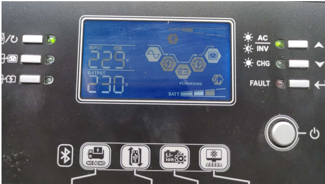
Fig 4.1 Home Screen of Axpert showing the battery icon (flashing when communication is normal) and the SoC bar reflecting 25% increments of the battery SoC)
