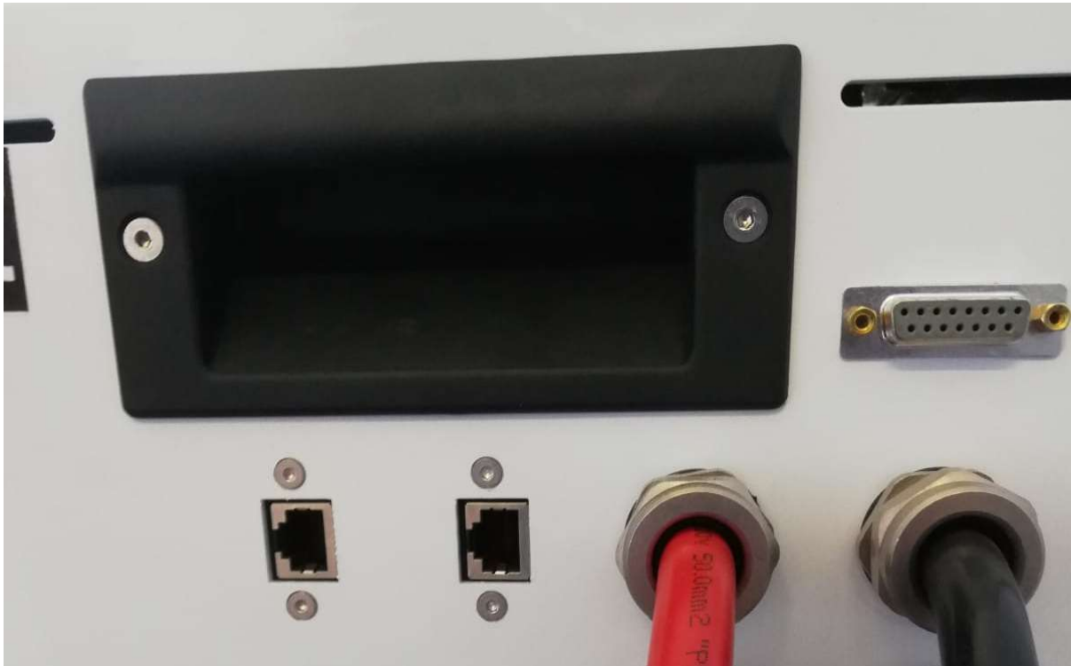
Figure 5.2 Picture Showing 2 x RJ45 Sockets for CAN Bus (DB15 Plug shown here for Analogue and Relay Control is not available in new models)
